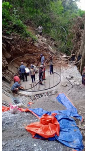
Building Water Tank
